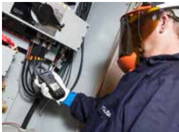
Analyze Power-related Issues
